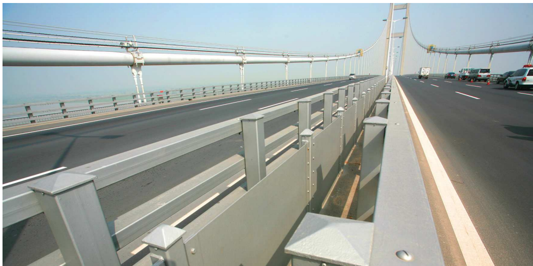
Figure 3: Central stabilizer mounted on the deck of Jiangsu Runyang Bridge
